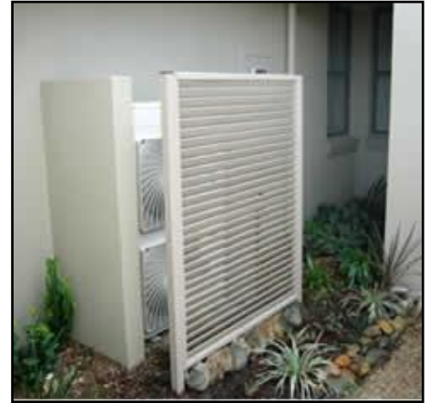
An example of an air-conditioning screen located at ground level (Sourced from: spec-net.com.au )
