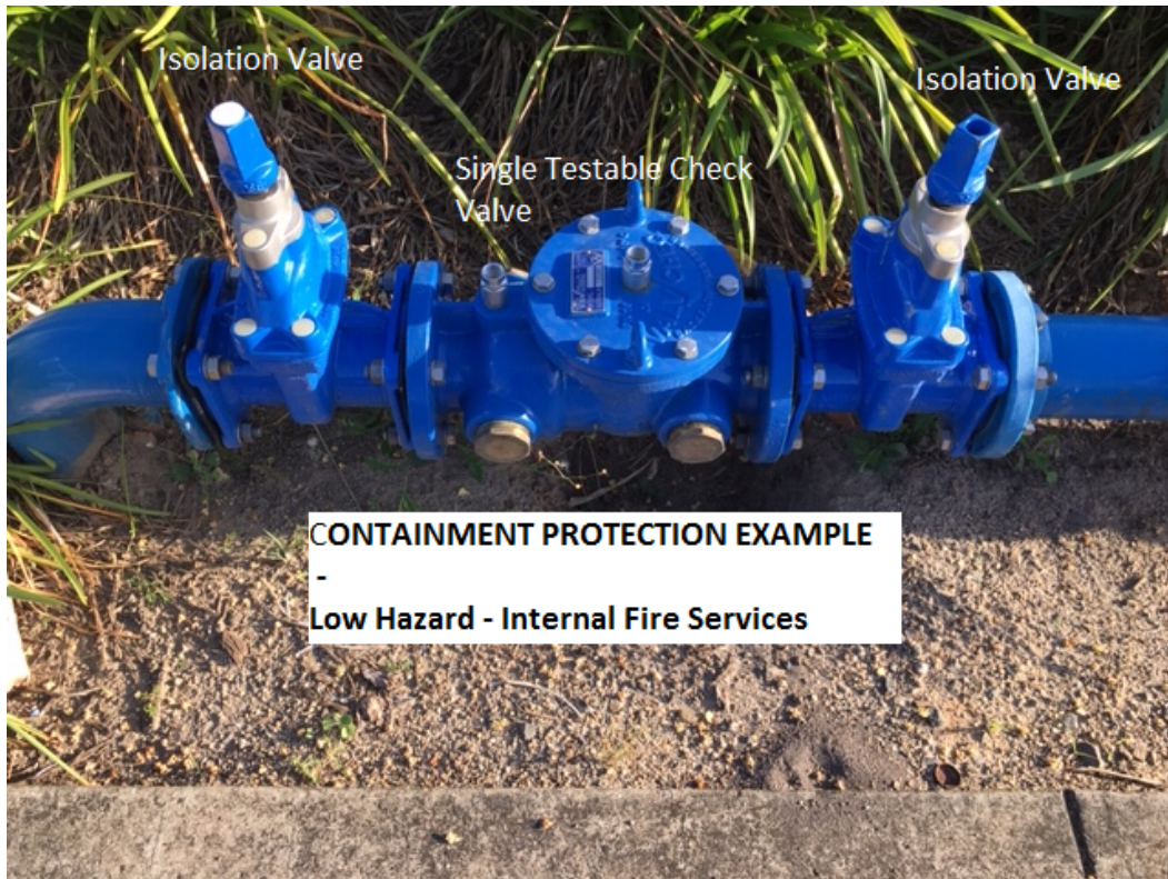
Picture 3 :Low Hazard Containment Protection – Single testable check valve (In this instance internal devices have individual and zone protection.)
