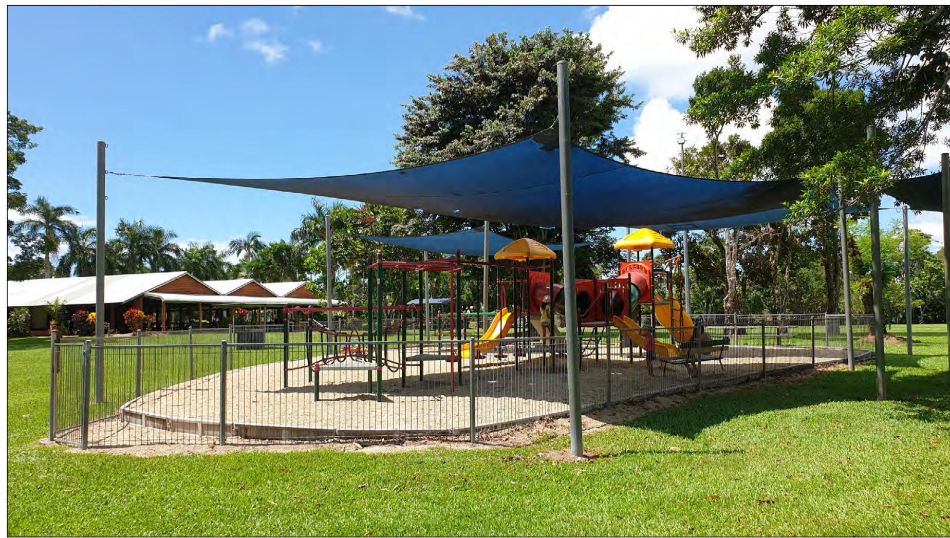
Existing playground is dated and old style. It needs rubberised soffit under.
