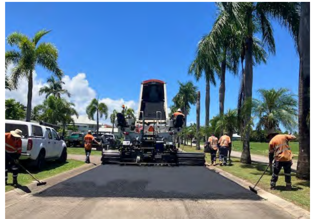
Caption: Road reseal being undertaken as part of the Port Hinchinbrook Normalisation Project.
